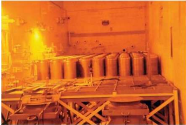
Source: West Valley Demonstration Project. High-level waste canisters in a shielded room at the West Valley Site (viewed through protective glass).
