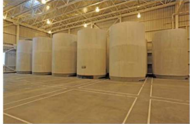
Source: Naval Nuclear Propulsion Program. Navy's spent nuclear fuel canisters surrounded by protective concrete overpacks in a storage building at DOE's Idaho site.
