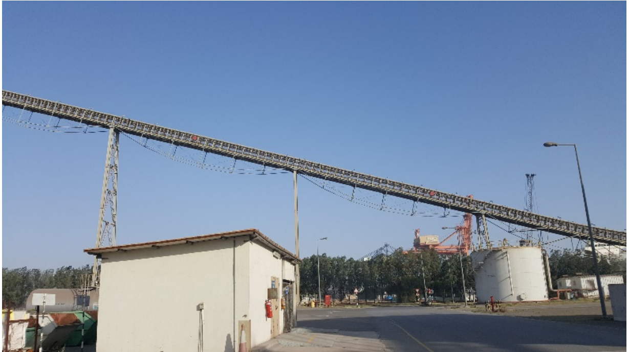
Overhead Conveyor – sprinkler-protected Courtesy of SOHAR Aluminium LLC
