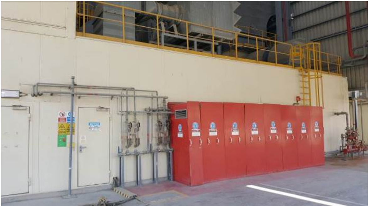
Adequate Fire Protection of GTs
