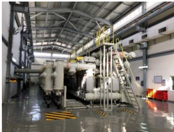
SF6 insulated busbar systems (GIS)
