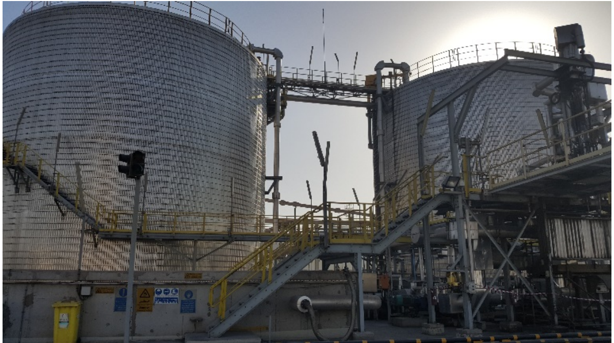
Pitch Tank – Adequately spaced and protected Courtesy of SOHAR Aluminium LLC
