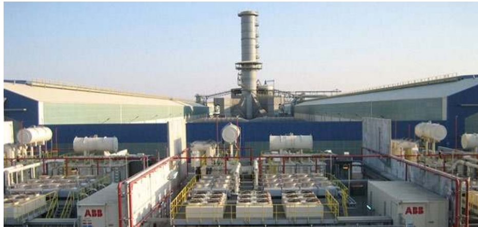
Main Substation RTs
