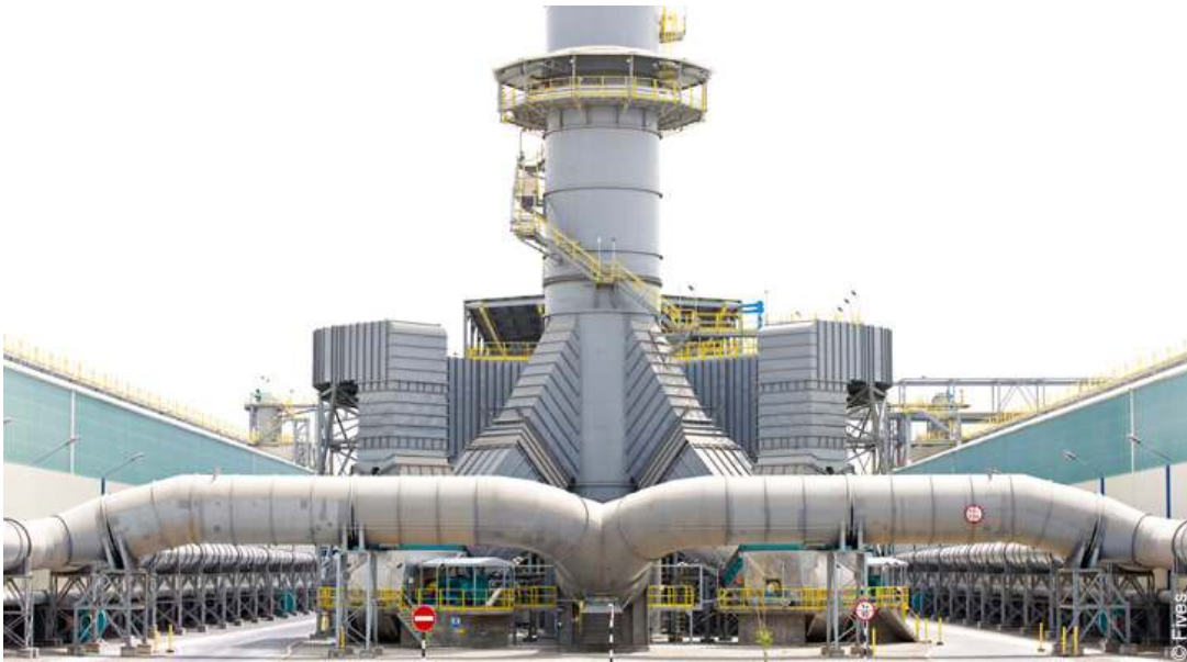
Gas Treatment Center - Courtesy of SOHAR Aluminium LLC
