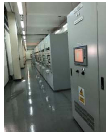
GIS Bay Cabinets
