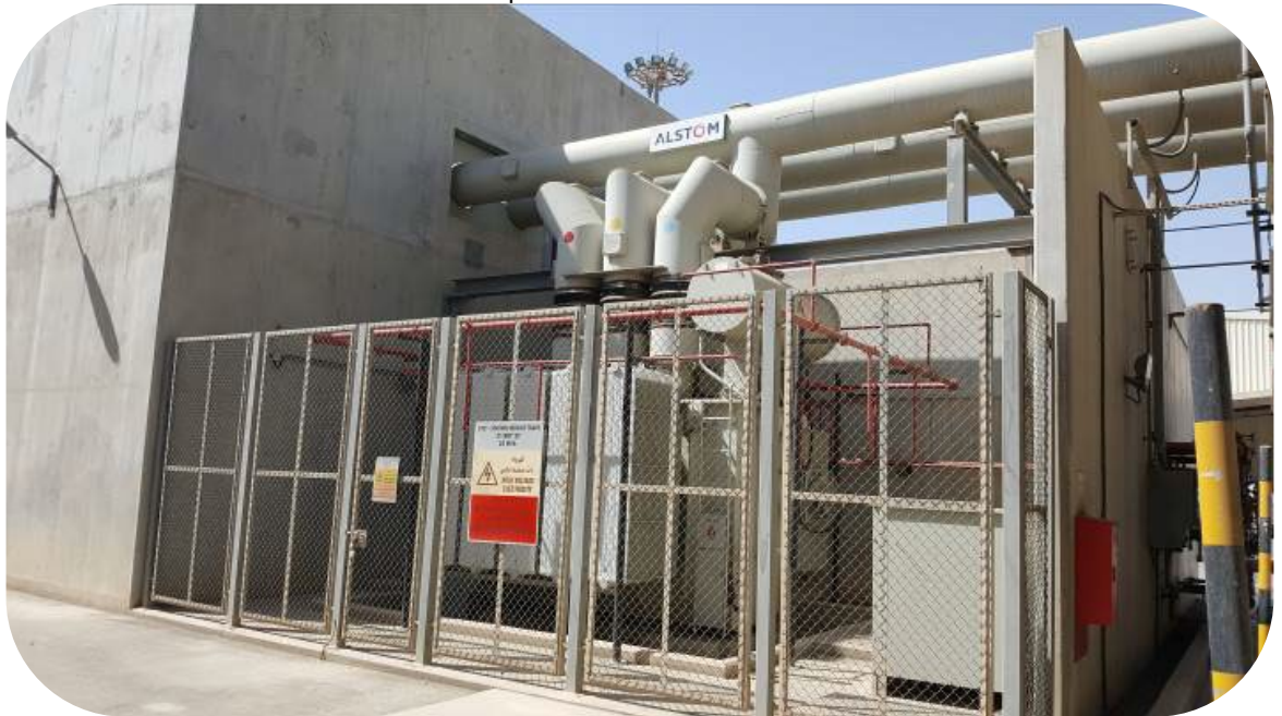
Adequate Segregation & Fire Protection of Oil-Filled Transformers Courtesy of SOHAR Aluminium LLC
