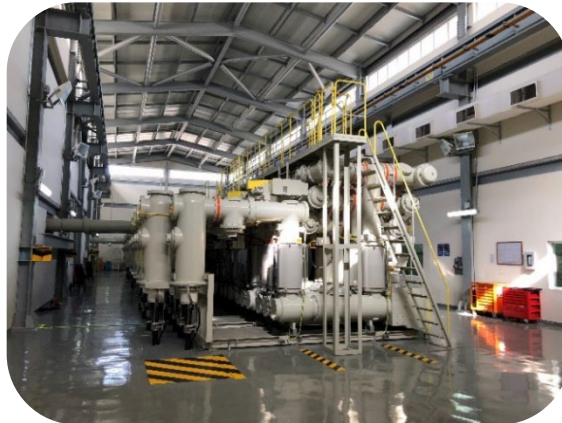
SF6 insulated busbar systems (GIS)
