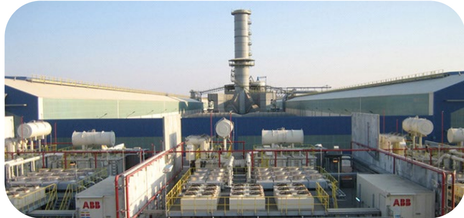
Main Substation RTs
