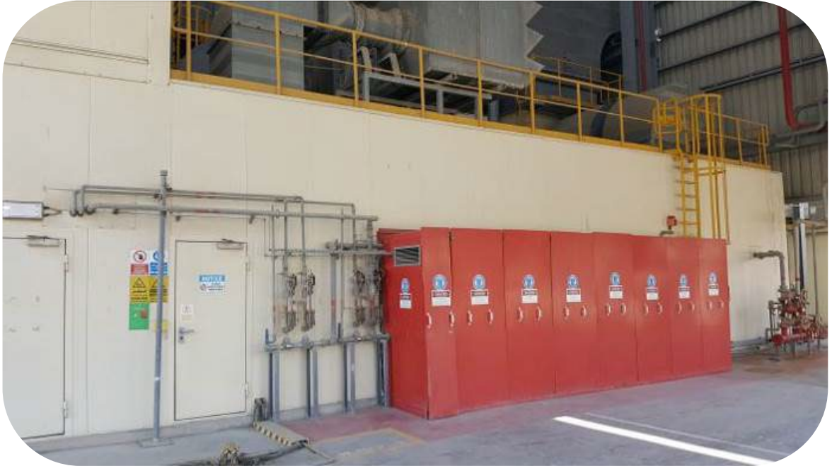
Adequate Fire Protection of GTs
