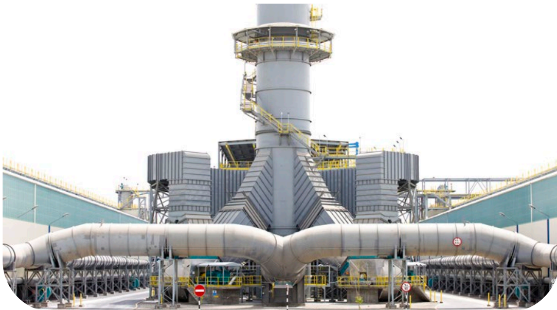
Gas Treatment Center—Courtesy of SOHAR Aluminium LLC
