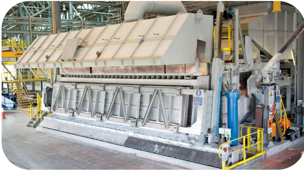
Cast House furnace—Courtesy of SOHAR Aluminium LLC
