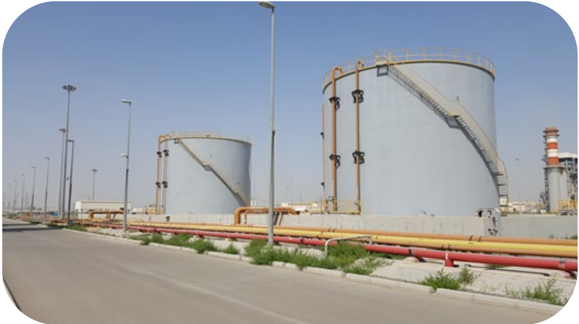
Fuel oil tanks adequately spaced and secondary retention provided Courtesy of SOHAR Aluminium LLC—Captive Power Plant
