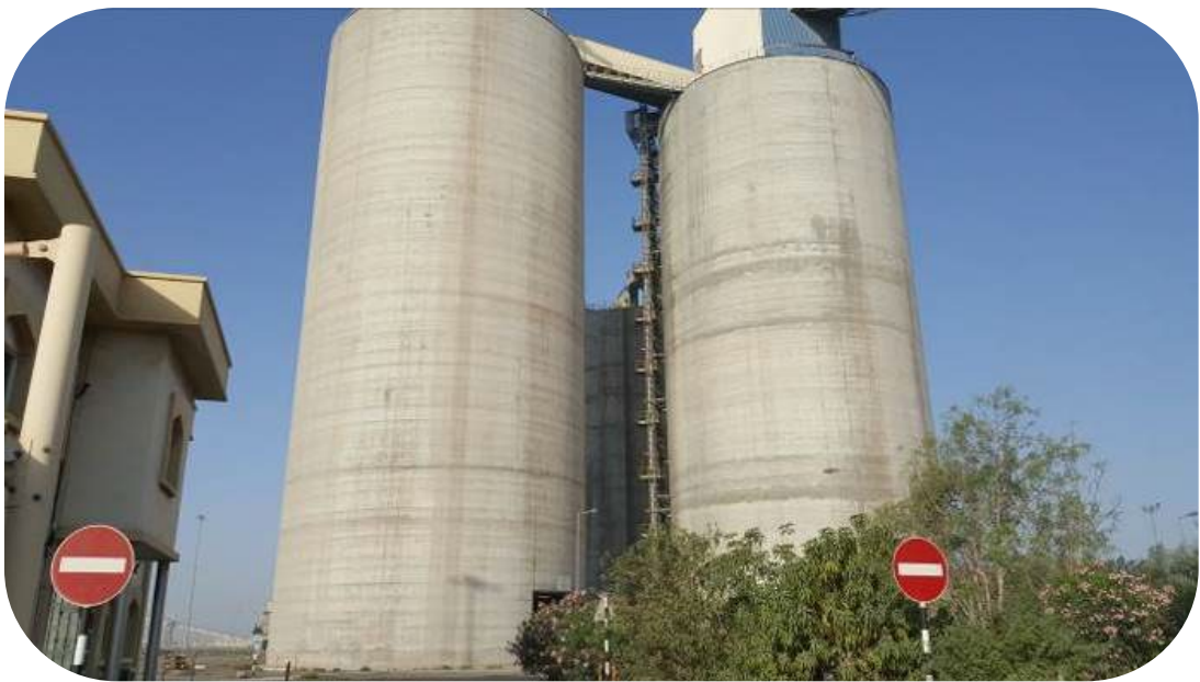
Alumina silos Courtesy of SOHAR Aluminium LLC
