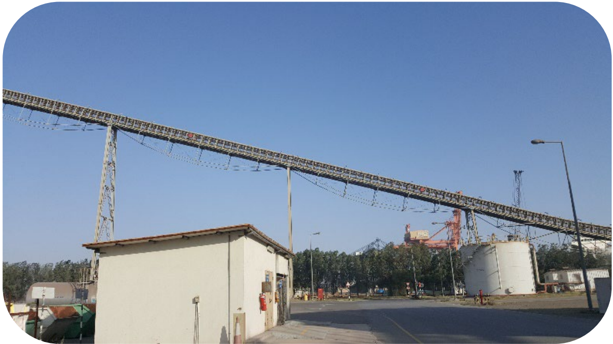
Overhead Conveyor—sprinkler-protected Courtesy of SOHAR Aluminium LLC
