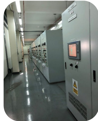
GIS Bay Cabinets
