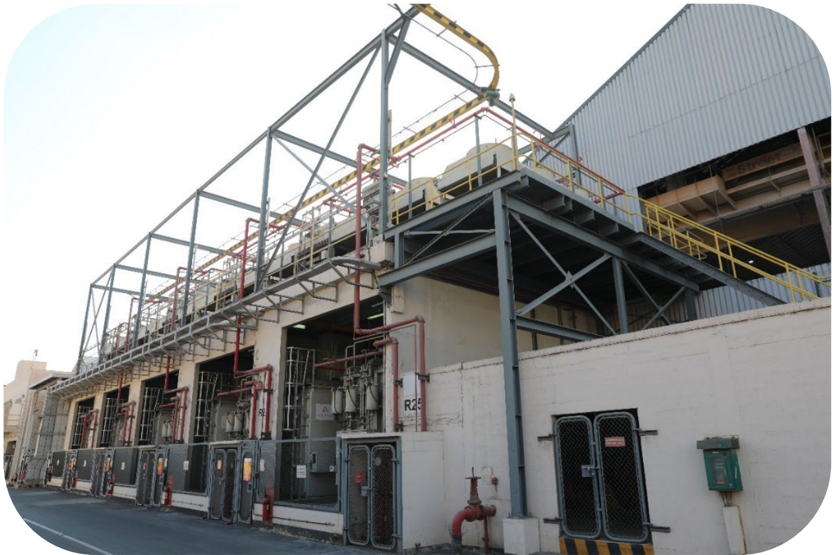
Well segregated & sprinkler-protected transformers Courtesy of Aluminium Bahrain B.S.C. (Alba)
