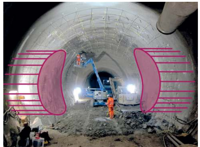
FIGURE 4: INSTRUMENTATION OF CROSSRAIL LIVERPOOL STREET STATION CONCOURSE TUNNEL, SHOWING FIBRE OPTIC SENSORS BEING INSTALLED IN THE THICKENED LINING, WITH THE LOCATION OF THE FUTURE CROSS-PASSAGE EXCAVATIONS SUPERIMPOSED
