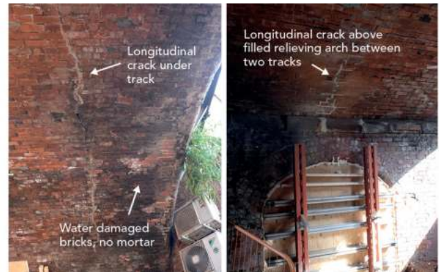
FIGURE 5: 150 YEAR OLD MASONRY VIADUCT SHOWING SIGNS OF DAMAGE
