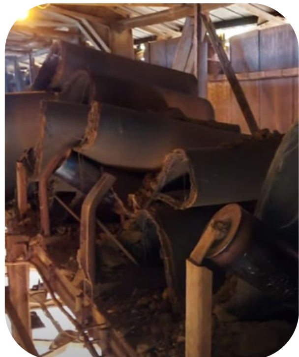
Belt conveyor snap due to joint failure
