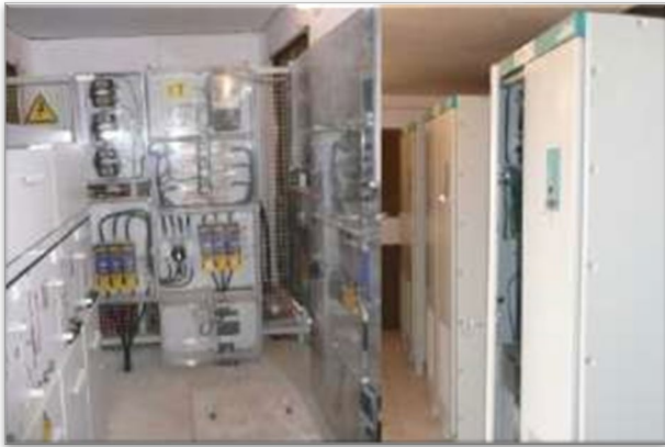
PV farm Substation
