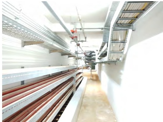
Integrated Steel Mill Main Substation (adequate sprinkler protection of the cable cellar)
