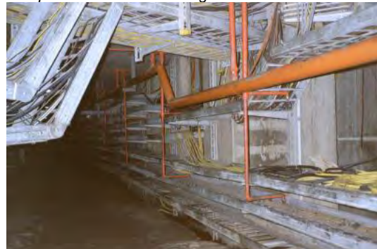
Inadequate Cable Tunnel Sprinkler Protection
