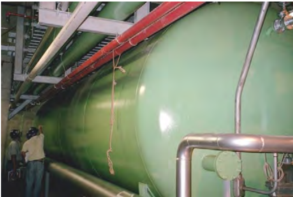
Underground lube oil reservoir
