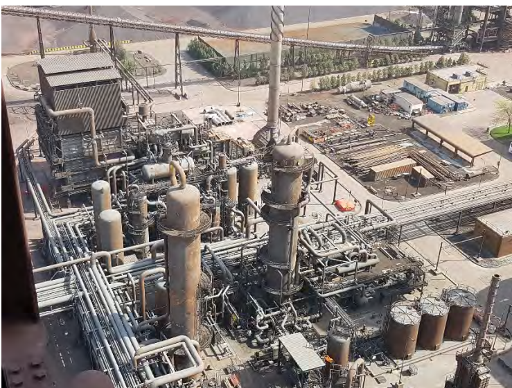
Natural Gas Reformer area
