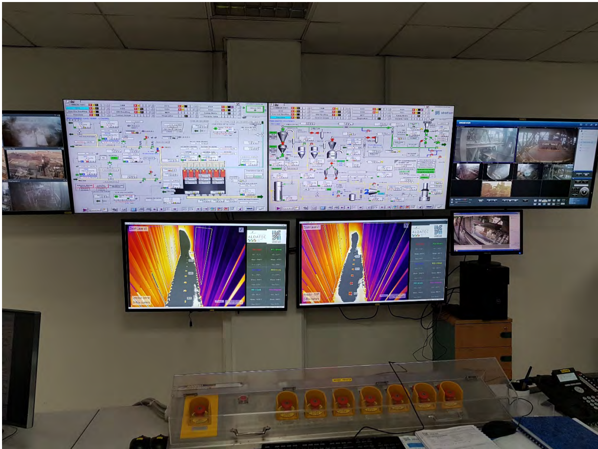
DR Control Room with PGH temperature monitoring system
