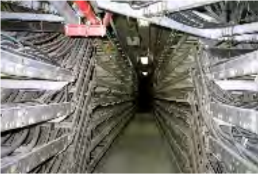
Unprotected Cable Tunnel
