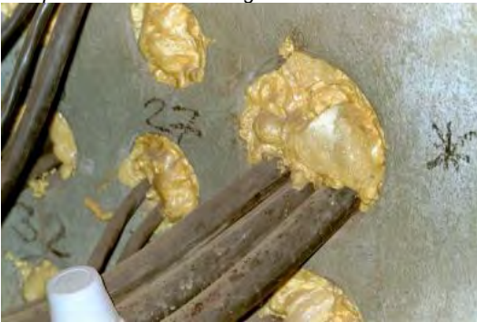
Inadequate Cable Sealing (PU Foam)
