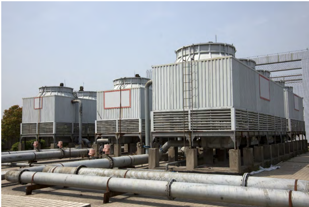
Cooling Tower with inside plastic fins
