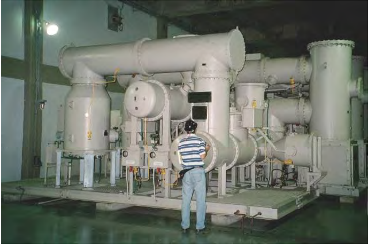
SF6 gas-insulated circuit breakers in a cut-off room
