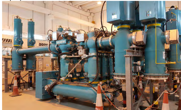
Integrated Steel Mill Gas Insulated System
