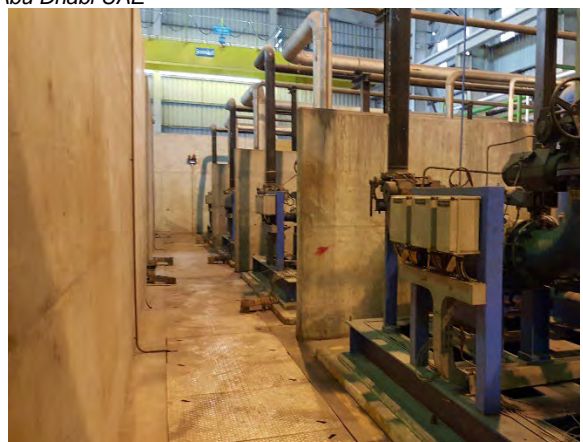
Oxygen compressors adequately separated by blast-resistive walls.
