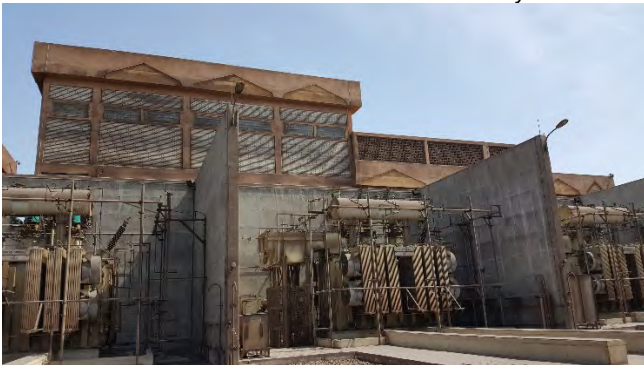
National Grid Substation (back) supplying Integrated Steel Mill Transformers (adequate passive and spray protection)
