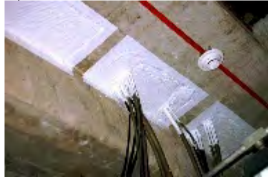
Adequate Floor Cable Sealing
