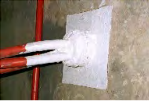
Adequate Wall Cable Sealing
