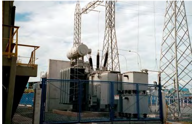
Inadequately separated oil-filled transformers
