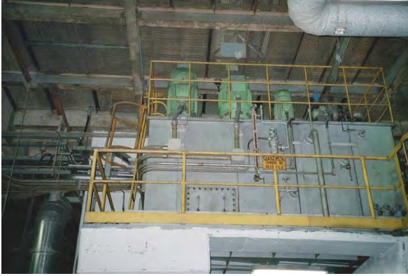
Overhead lube oil reservoir
