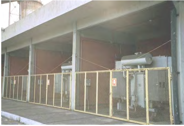
Well-separated oil-filled transformers
