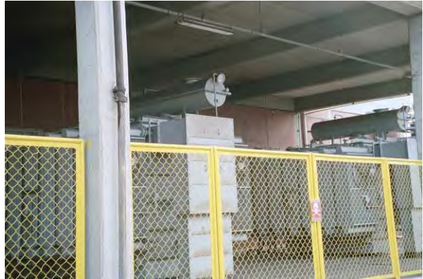
Inadequately separated oil-filled transformers
