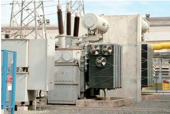
Well-separated oil-filled transformers
