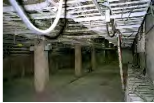
Unprotected Cable Vault
