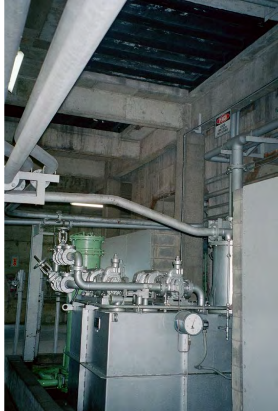
Aboveground lube oil reservoir
